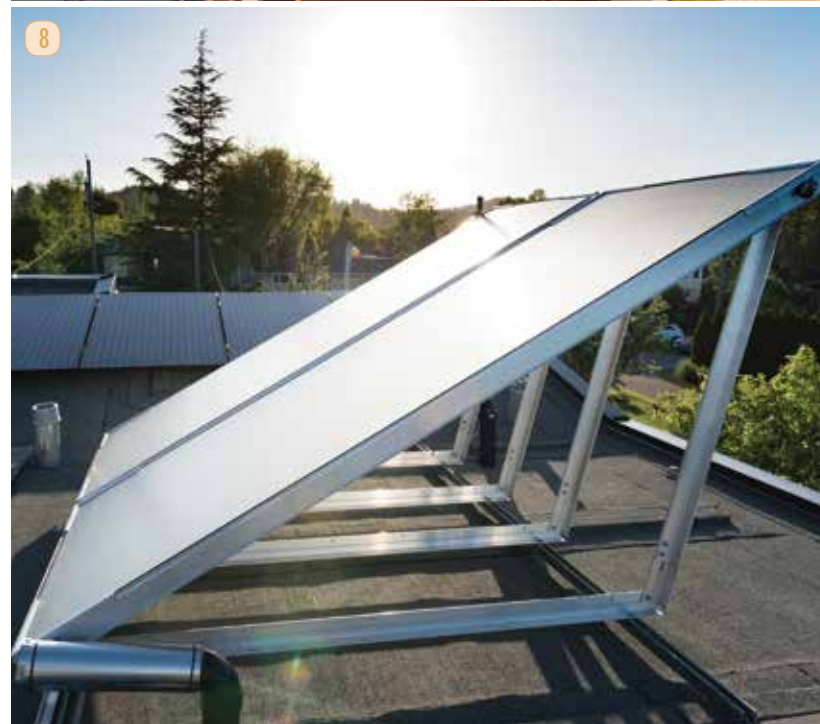
6 - Photovoltaic Panels. 7 - Easy access to roof for maintenance of PV array. 8 - Solar thermal domestic hot water system supplied by Viessmann .
